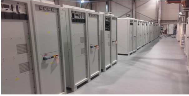
Fig. 35: Stored quadrupole power converters.
