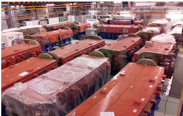
Fig. 33: Stored dipole magnets for HESR in Jülich.
